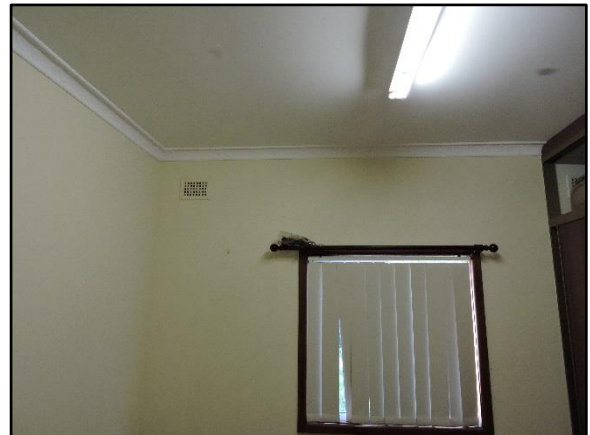
Figure 23. Ceiling of second bedroom.
