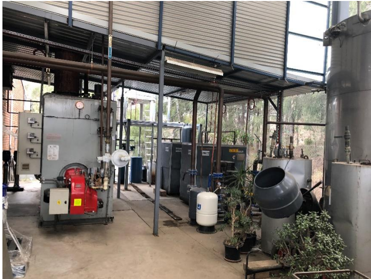
Exterior of laundromat building – boiler area.
